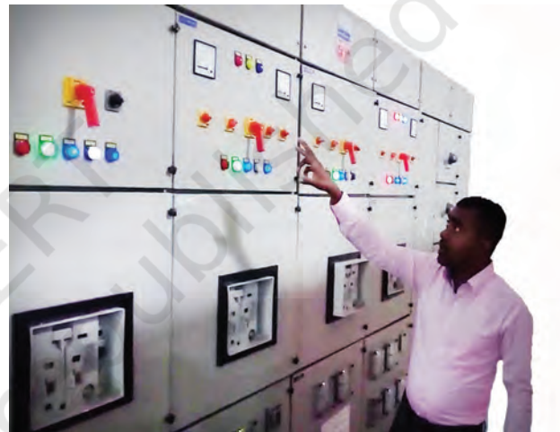
Fig. 1.44: Switchgear in the substation
