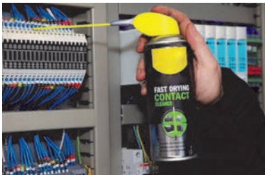
Fig. 11.7: Equipment cleaning spray
