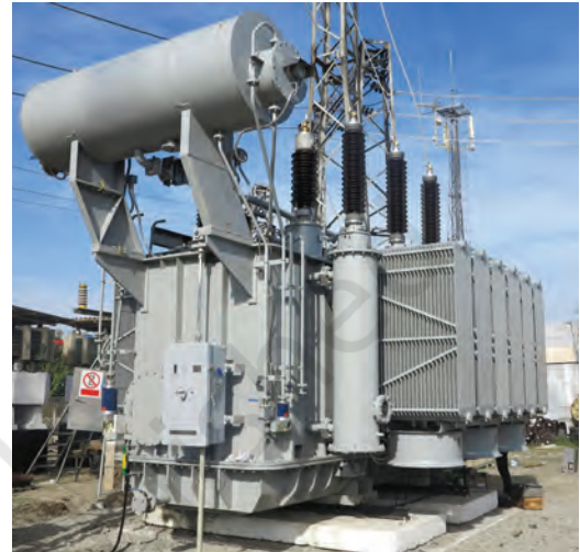
Fig.1.14: Transformer in the electrical substation
