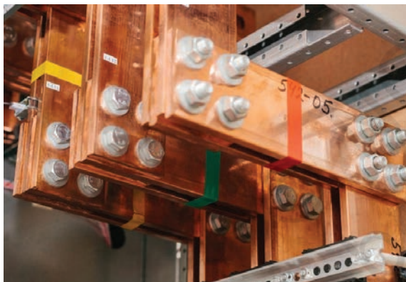
Fig. 2.12: A busbar for power distribution
