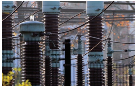
Fig. 10.2: Current transformer in an electrical sub-Station
