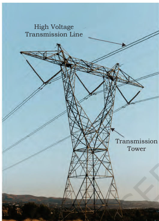
Fig.1.2: Transmission tower for transmission of electric power
