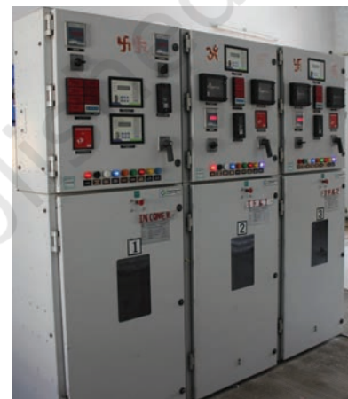
Fig. 5.5: Power panel board
